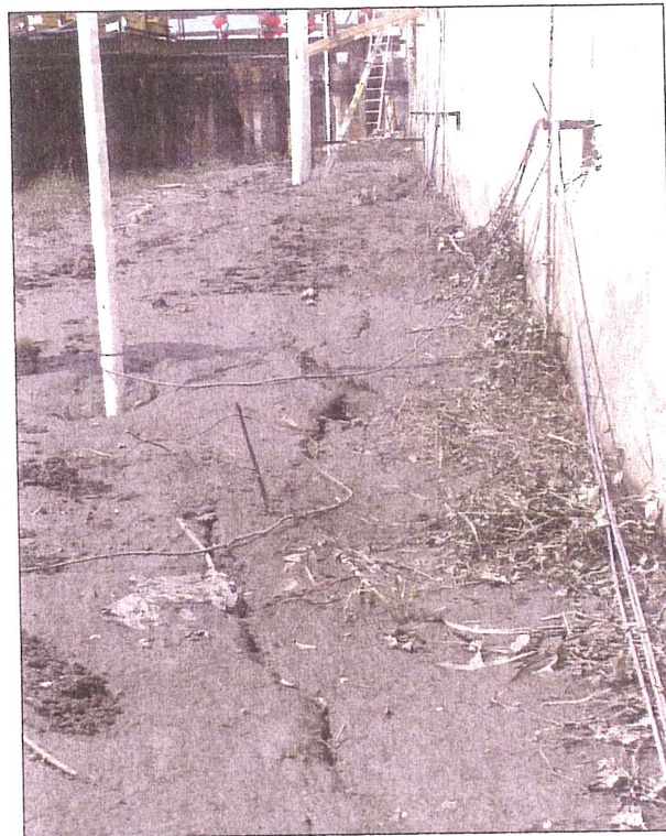
Figure 6.13 – Crack in Canal Side Embankment After Phase I Load Test.
