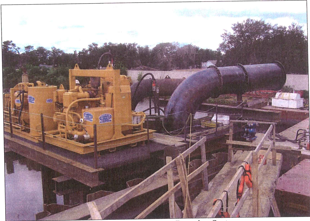
Figure 2.10 – Emergency Pumping System
